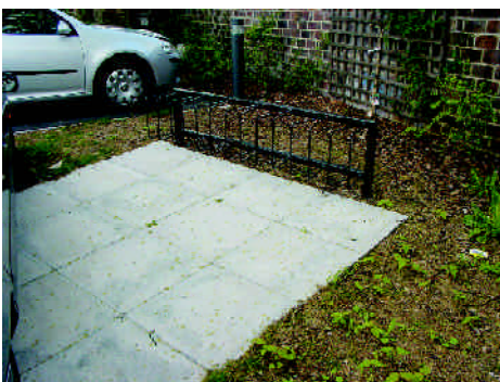
Cycle parking facilities for visitors should be provided alongside visitor parking spaces and kept accessible at all times. The surrounding areas of landscape should be easily accessible for maintenance, unlike in this photo.
